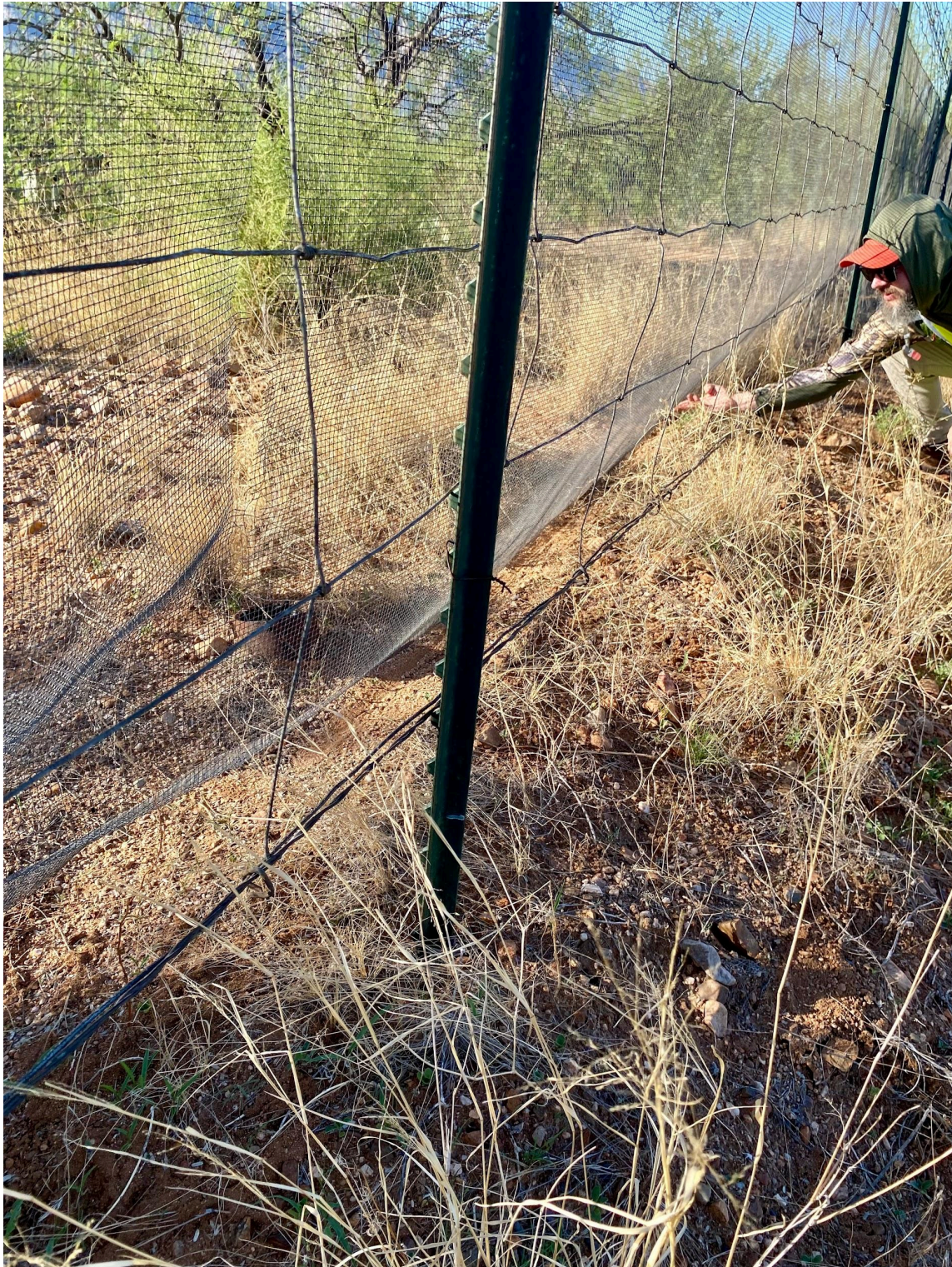
Mesh footing has come loose allowing animals to push through or crawl under the fenceline at 32.452782, -110.932226. Needs reburied.
