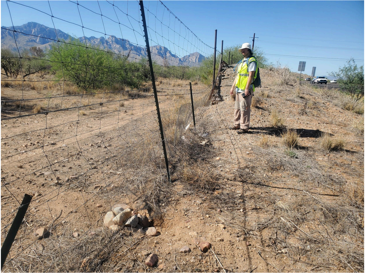
Northbound fence line located at 32.472264, -110.923503, collision damage to fence and posts that had been patched back together. One smaller opening was partially repaired with rocks.
