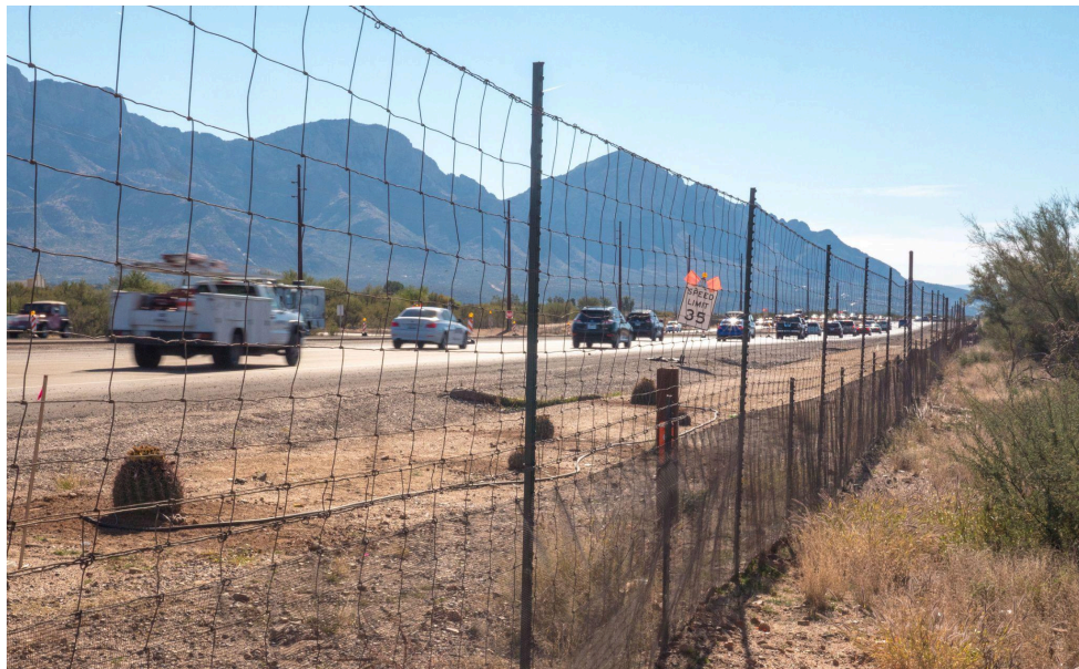
Above: The wildlife funnel fence when first installed in 2016.
