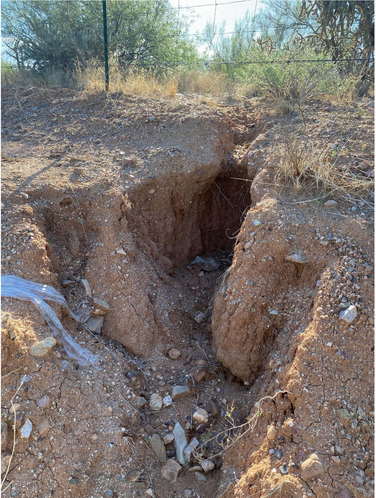
Erosion caused this opening, located at 32.452782, -110.932226.
